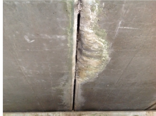
spalling under slab 2
